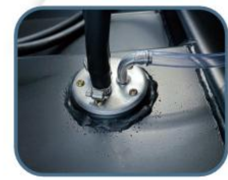
Fuel inlet and return pipe
